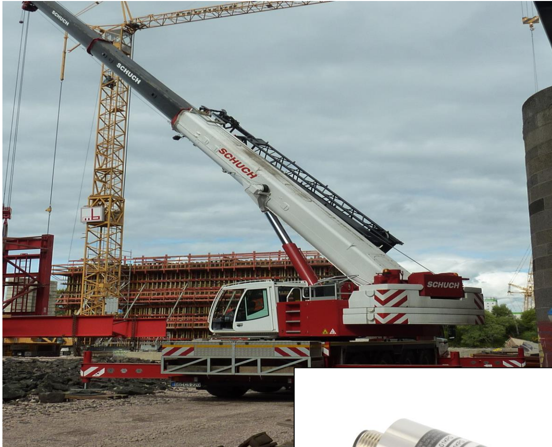
Figure 1: construction vehicle with a hydraulic lifting system on the new Rhine bridge building site between Mainz and Wiesbaden.
